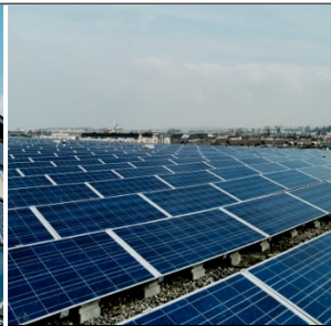
PV power plants
